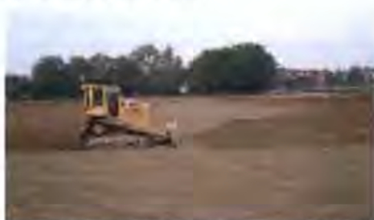
To create a level surface, it may be necessary to strip the topsoil, regrade the subsoil, and replace the top soil
