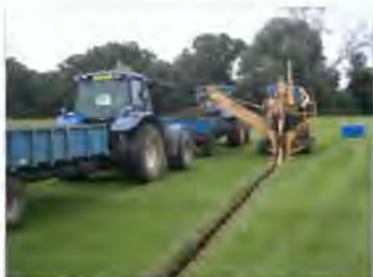
Drain installation normally requires the use of specialist trench machinery fitted with laser guidance
