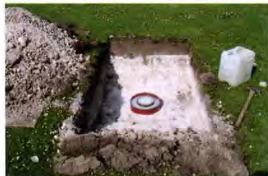
An investigation of the infiltration on the site is necessary to inform the design of the natural turf facilities
